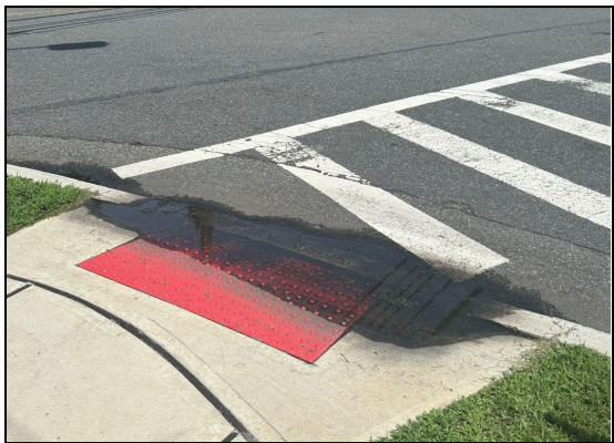
Figure 46: Misaligned Dome Pad and Puddle
