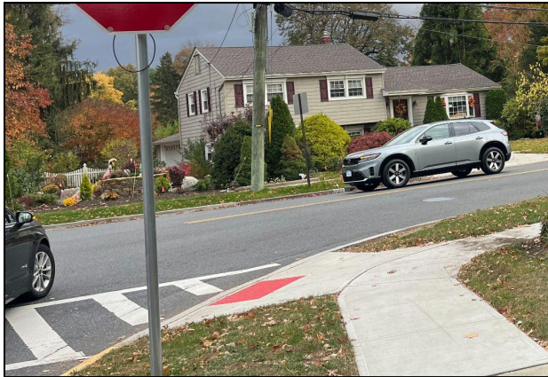
Figure 14: Truncated Dome Plate Misaligned
