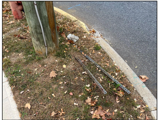
Figure 11: Crumbling Curb and Metal Posts
